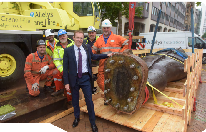
Mayor of the West Midlands, Andy Street, joining the team assisting in the removal of the city's iconic Iron Man, which marked the kick-off of tram extension works in Birmingham.
